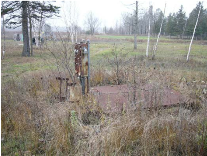
Figure 6.5. Pumping station at Sugar Shack Lagoon.
